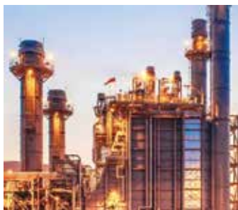
Power Utility Industries
